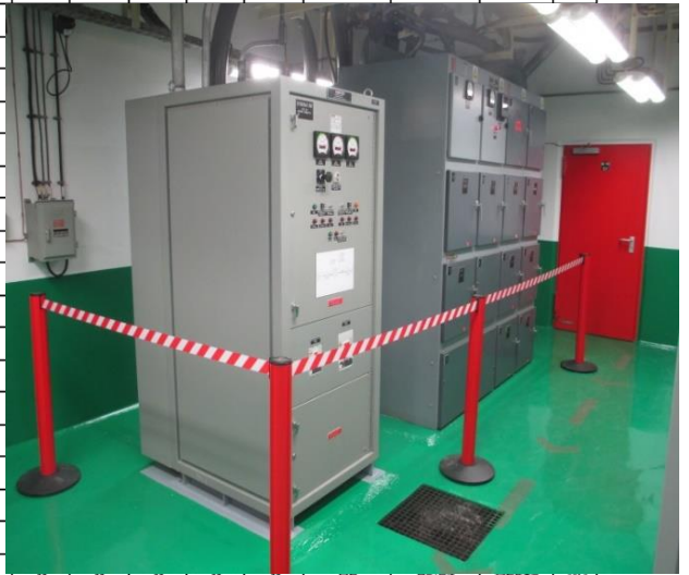
Figure 9 - List of the protected equipment by SD phase and an example how the protected equipment is marked
