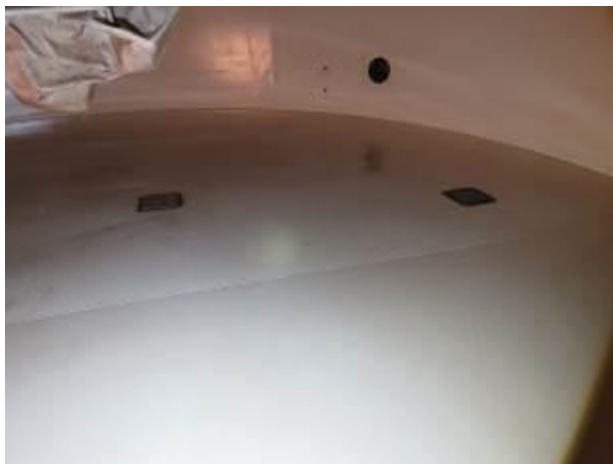
Figure 14: Steel plates inside CY tank
