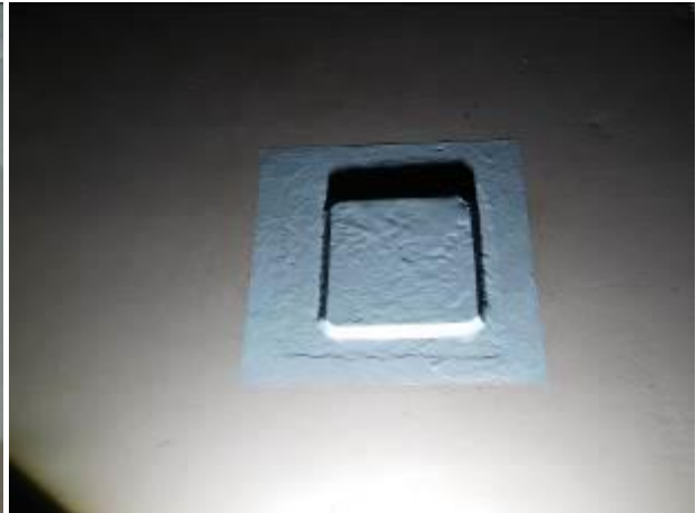
Figure 13: Coated steel plate inside CY tank
