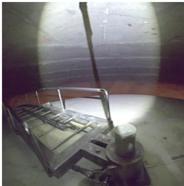
Figure 11: Rotating ladder for the top of the dome access. The original ladder was replaced with a new one in 2021 to provide safer access.
