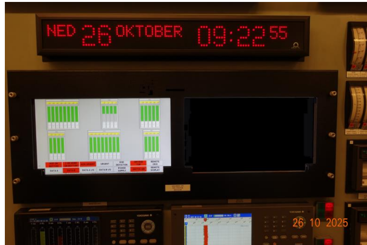
Figure 4: Single Display Failure
