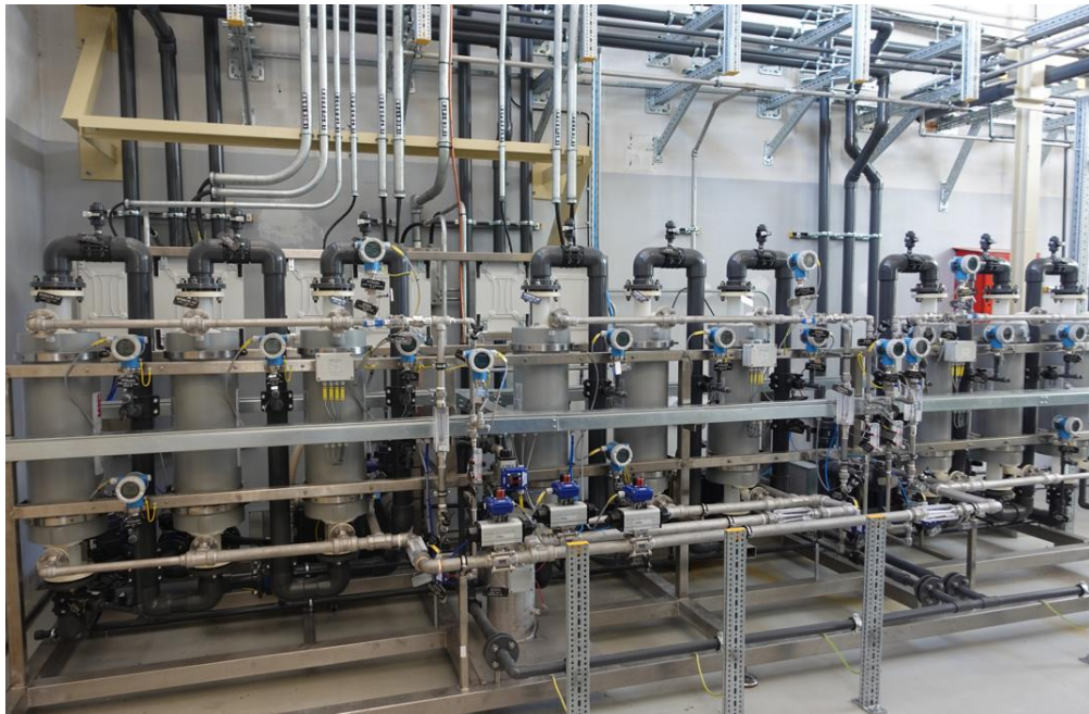
Figure 6: Gas Transfer Membranes
