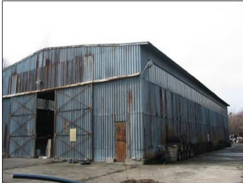
Figure 2: View of hangar H1 from the direction of hangar H2 - before the installation of pedestrian doors
