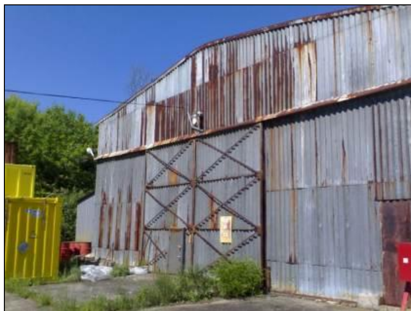
Figure 3: View of the front door hangar H1, after installing the pedestrian door
