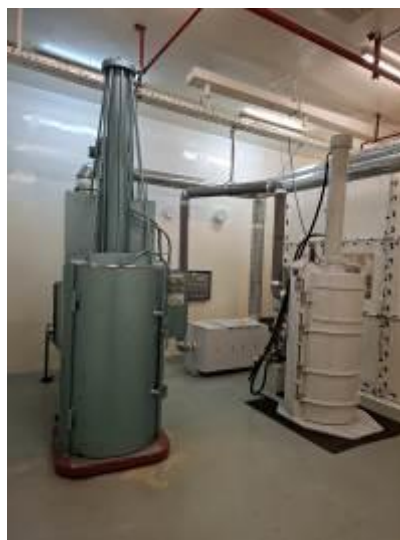
Figure 18: Compactors for RW in-drum compacting and compacting empty drums
