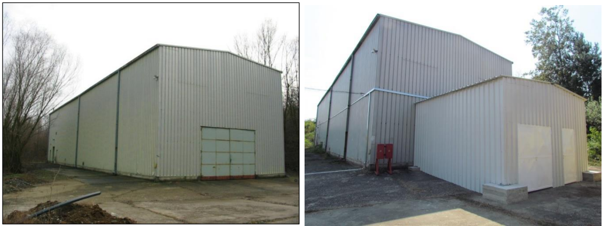
Figure 6: a) Photos of hangar H2 before b) after adding the assembly-disassembly structure at the material inlet and outlet
