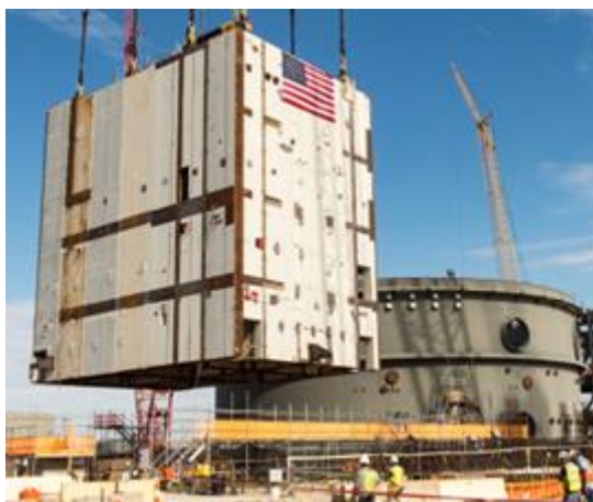
Figure 1: Installation of the CA20 module at Vogtle site (© Georgia Power Company All Rights Reserved)
